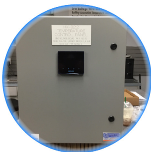
Watlow F4T Control Panel
