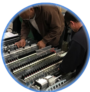
GTH Control Panels
